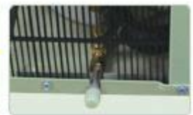
Cold tank drain
